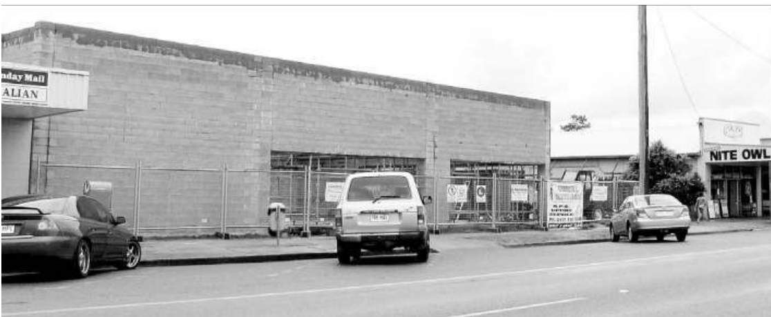
The site of the new IGA supermarket on Cartwright Street ... Construction is on track for its anticipated May opening
