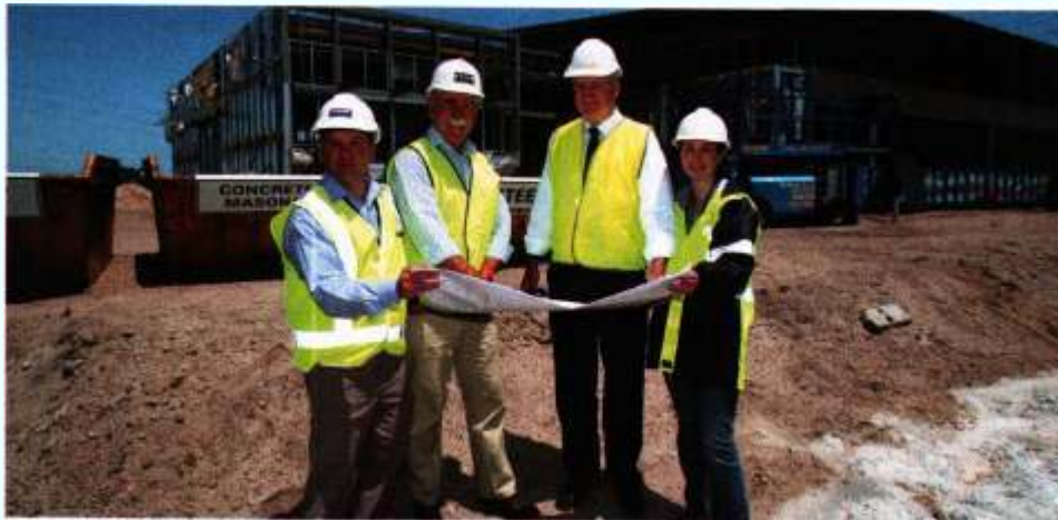
Candetti Constructions saved about 95% of material usually earmarked for landfill during its construction of the $6 million Maritime Skills Centre (MSC).
