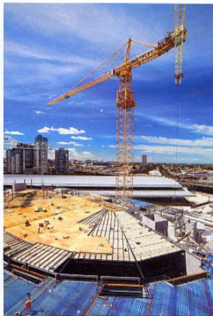
The largest tower crane ever erected in Australia is helping construct the new Melbourne Convention Centre.
