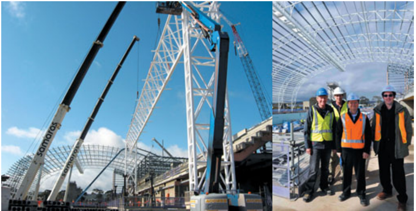
(L to R) Onsite during construction were Professor Roger Plank (Vice President, Institution of Structural Engineers UK), Matthew Gooding (SAC Project Manager, Candetti Constructions), Graeme Burmeister (Senior Structural Engineer, GHD), and Stuart Bater (Structural Engineering Manager, KBR).
