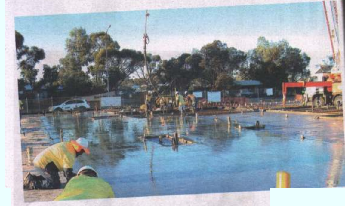
ABOVE AND LEFT: The second stage of the foundation slab for the new Roxby Police Station was poured and finished off in the early hours of last Thursday morning.
